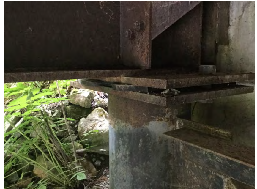
Right downstream bearing - typical all 4
