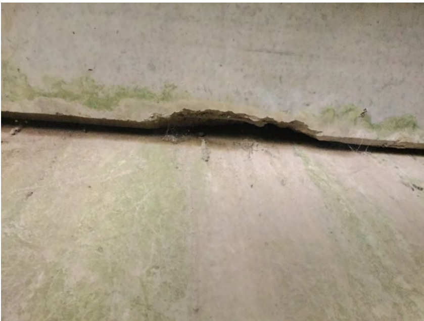
Damaged deck panel 1 on left approach
